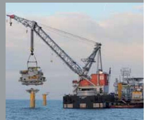
A substation being lifted onto its foundation from the barge Dina Launcher.
